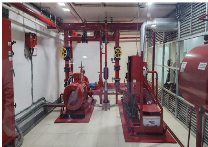
Fire Pump Room
